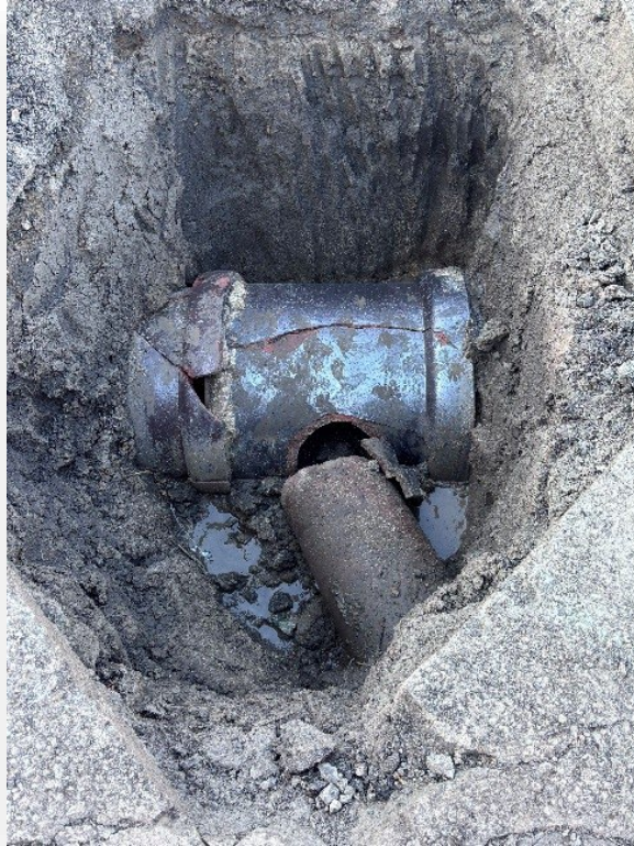
Storm sewer failure at NW 5th Street and Broadway. Aging underground infrastructure can remain out of sight until a failure requires immediate repair.
