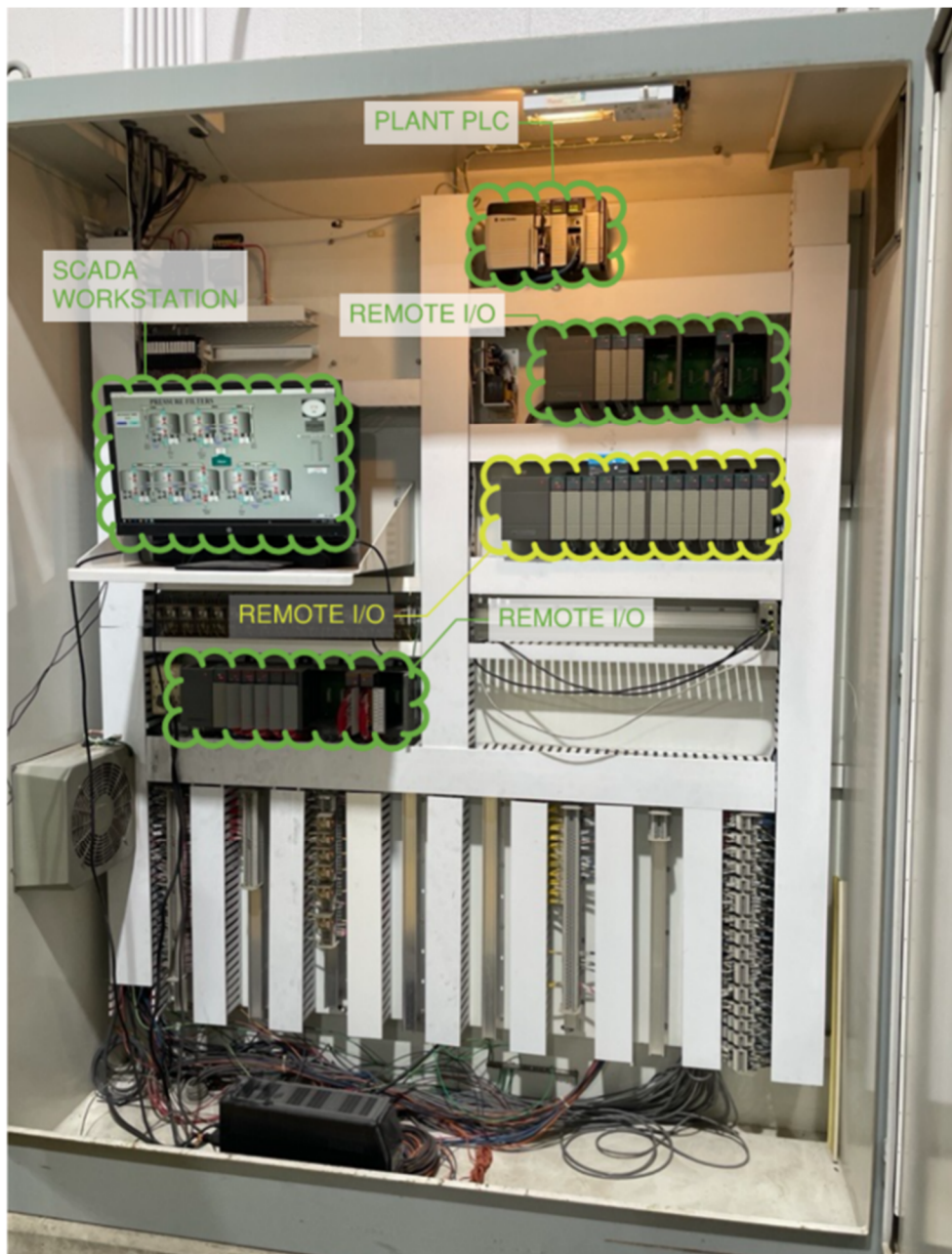
Figure 3: Plant PLC Cabinet
