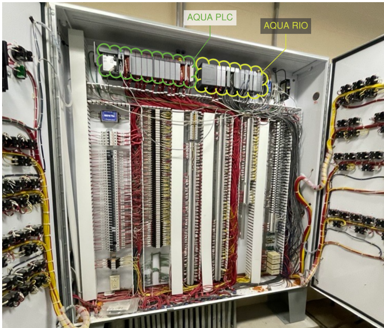
Figure 4: Aqua Vendor PLC Cabinet
