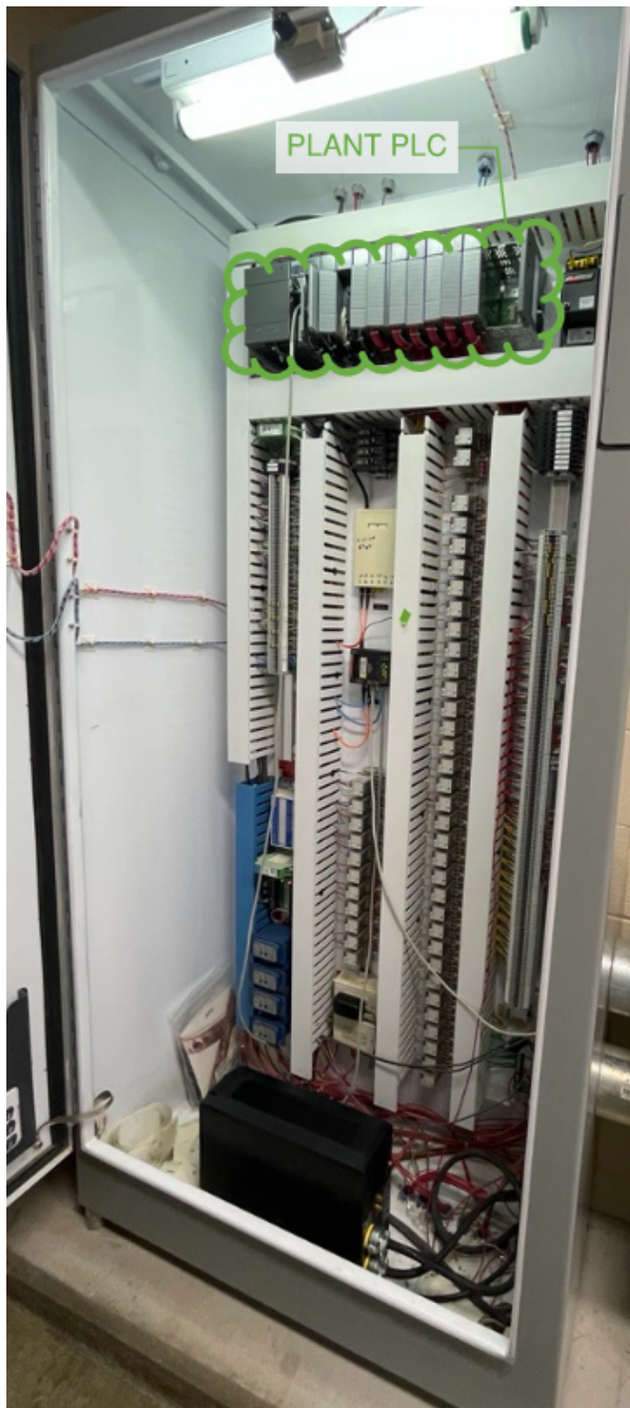
Figure 3: Plant PLC Cabinet
