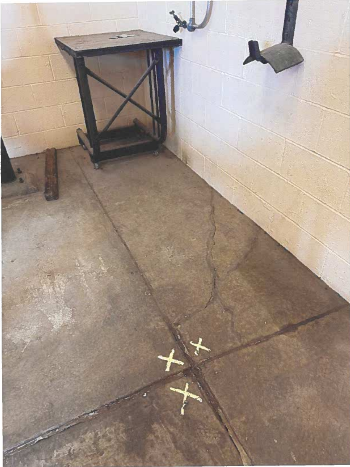
Figure 19: Cracks in concrete floor.
