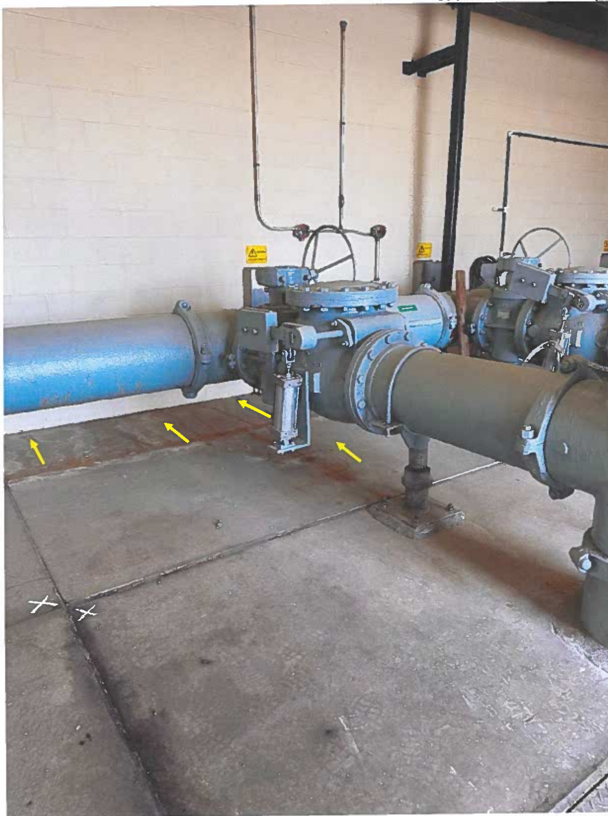
Figure 22: Note direction of staining on concrete floor.
