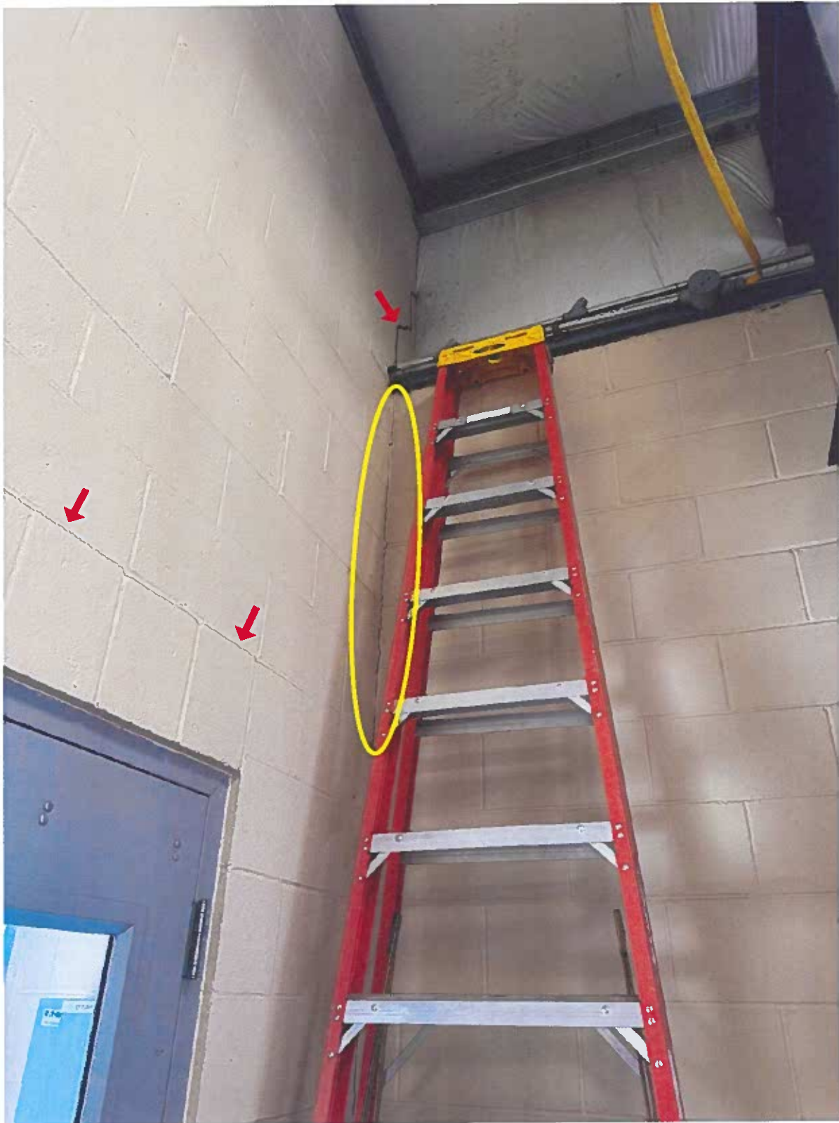
Figure 15: Separation at intersecting walls narrows and closes toward bottom.
