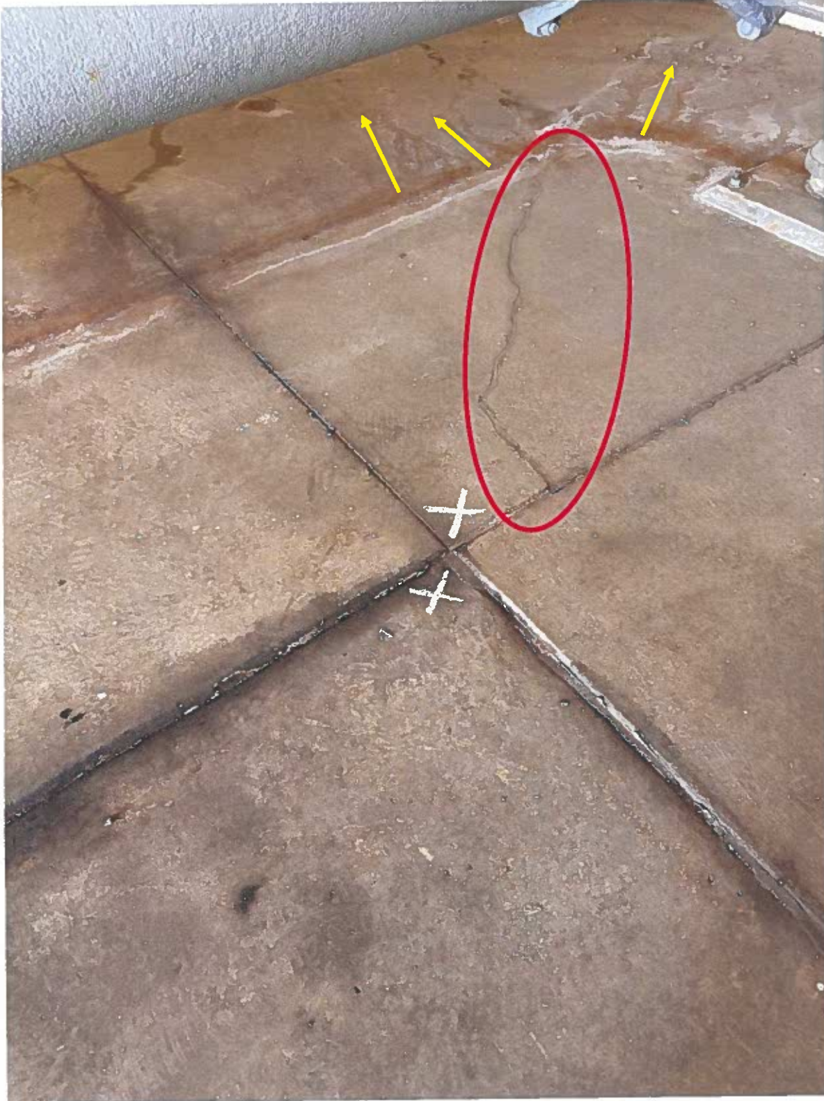
Figure 21: Cracks in concrete floor (appear to have previous repair). Note direction of water staining.
