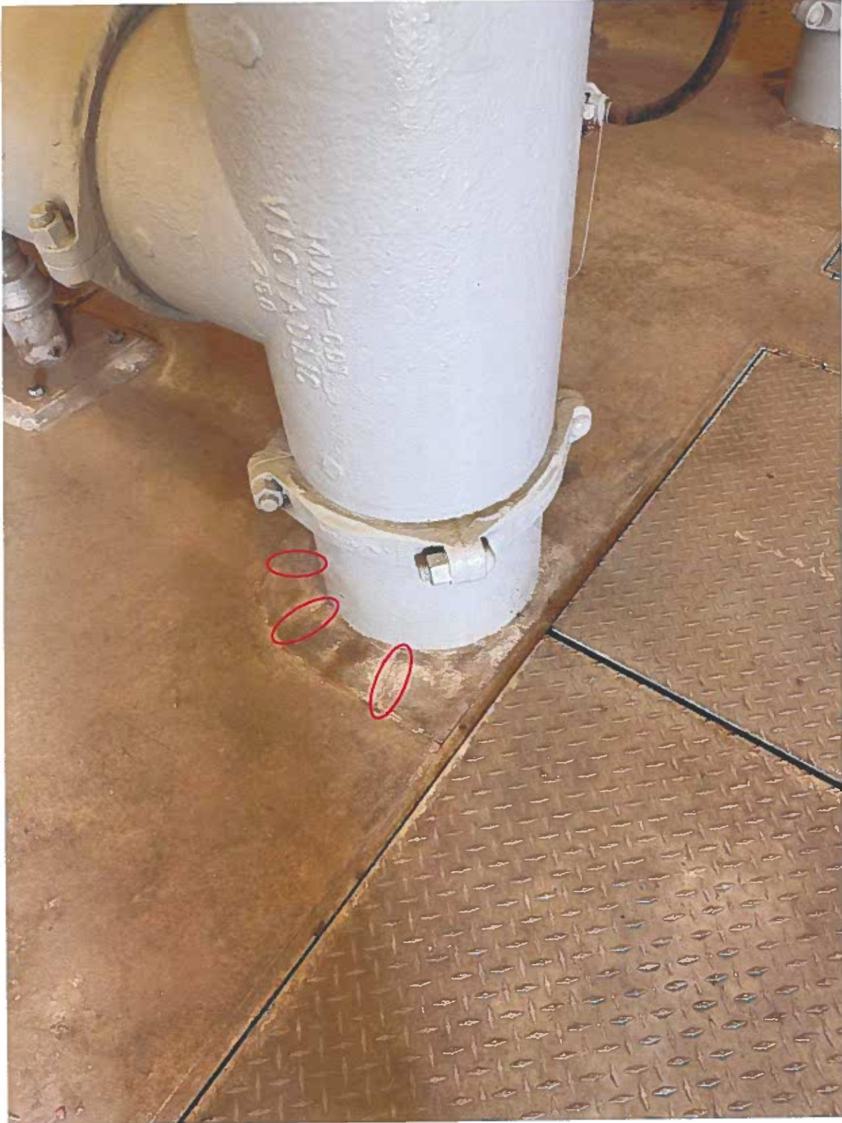
Figure 23: Cracks in grout around pipe penetration (typ.).
