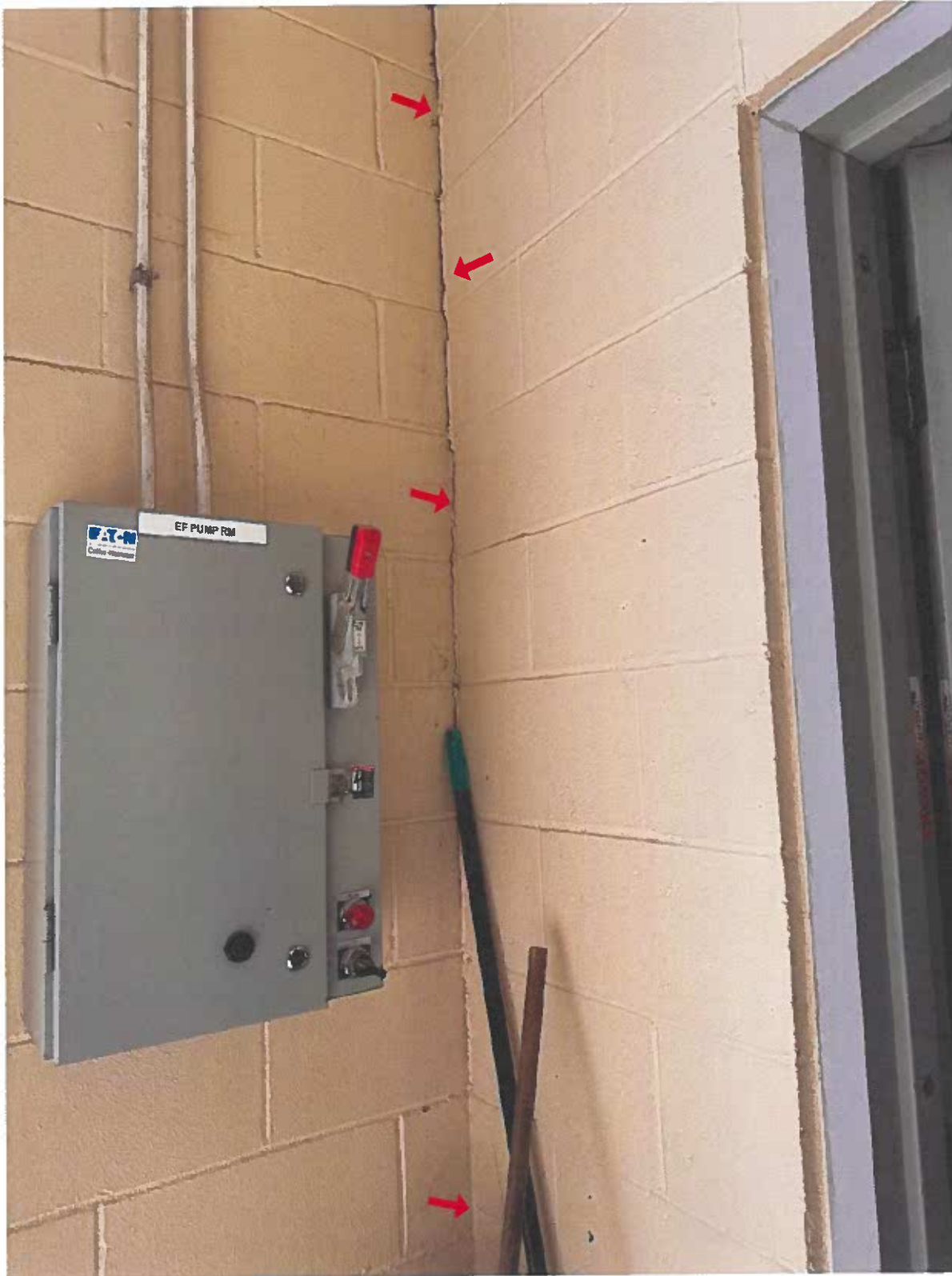
Figure 14: Separation at intersecting walls.
