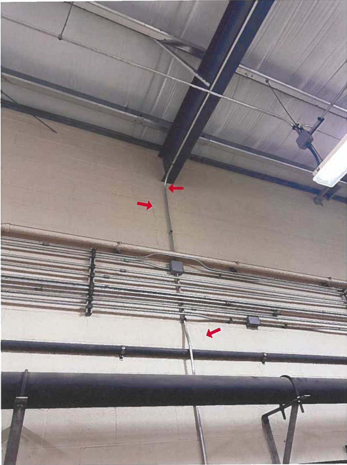
Figure 12: Cracks in masonry wall.
