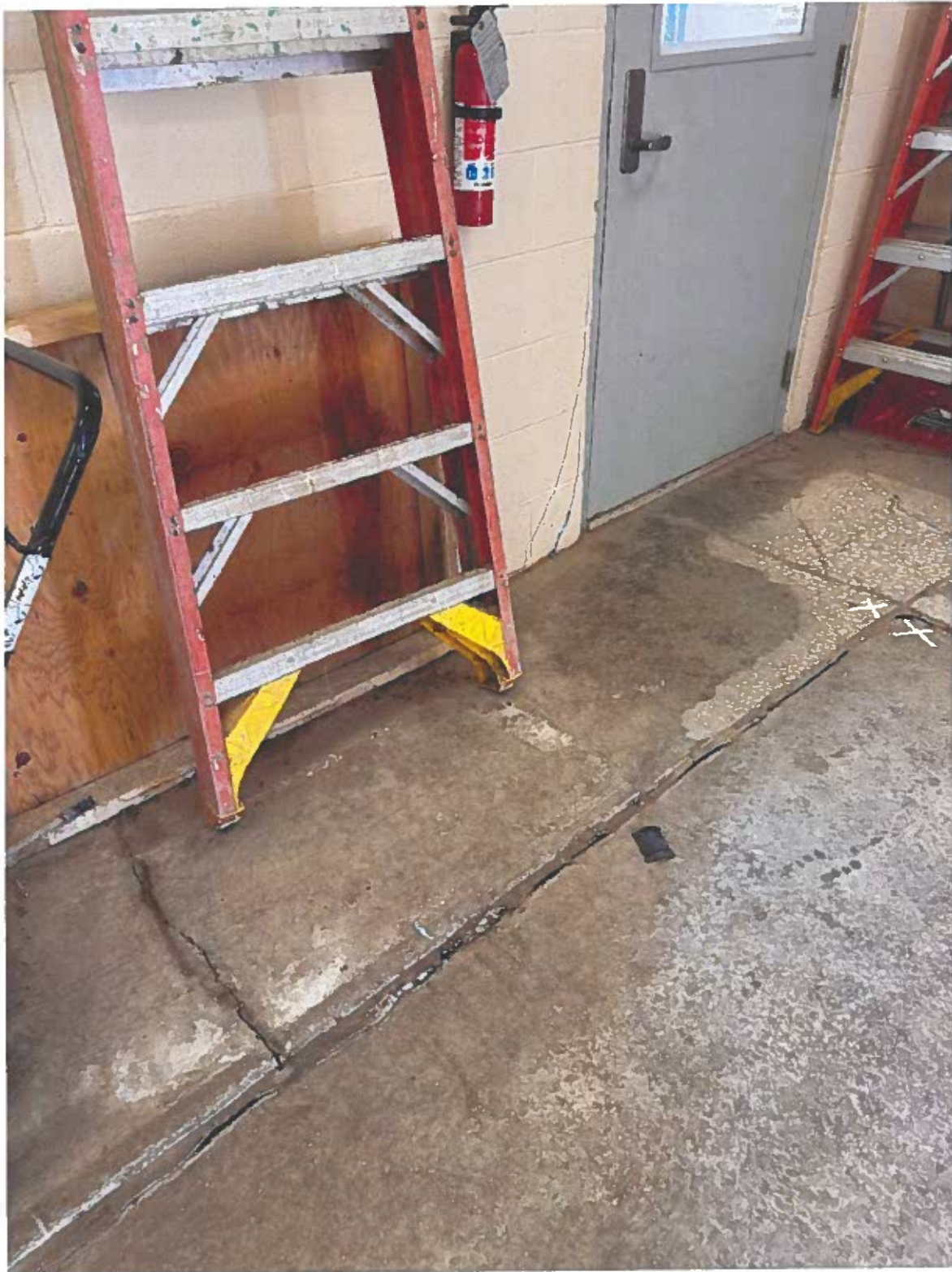
Figure 20: Cracks in concrete floor. Separation of sealant between Pump room concrete floor and deep well foundation.
