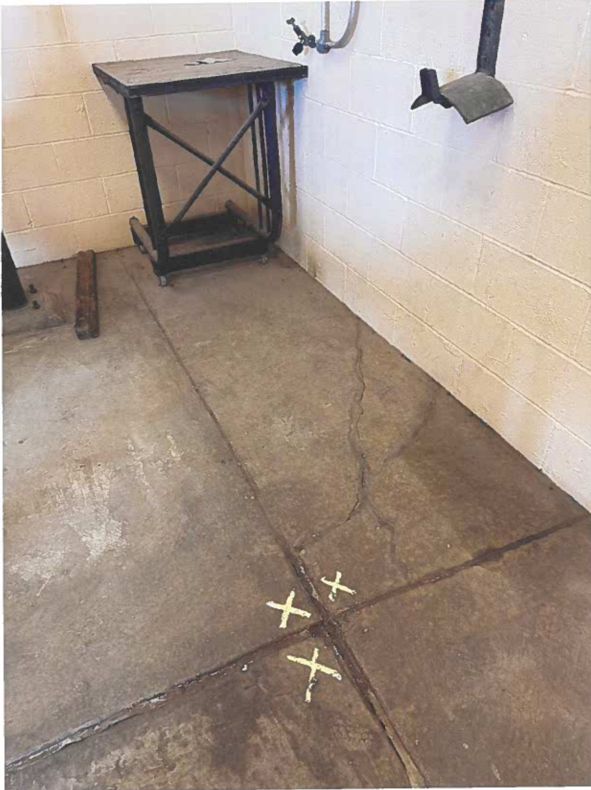
Figure 19: Cracks in concrete floor.
