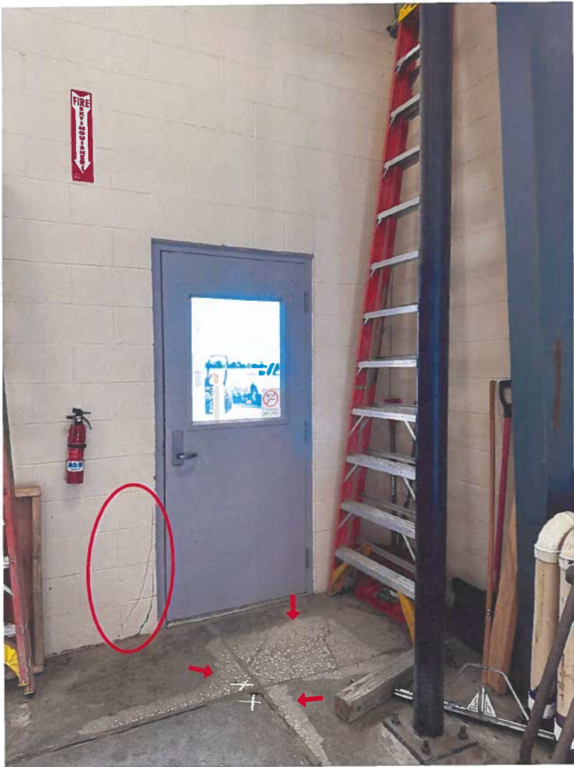
Figure 17: Cracks in masonry wall. Note purlin brace attached to CMU, frame penetration set in CMU, x-bracing penetrates CMU without space to move, and bridge crane attached to CMU.
