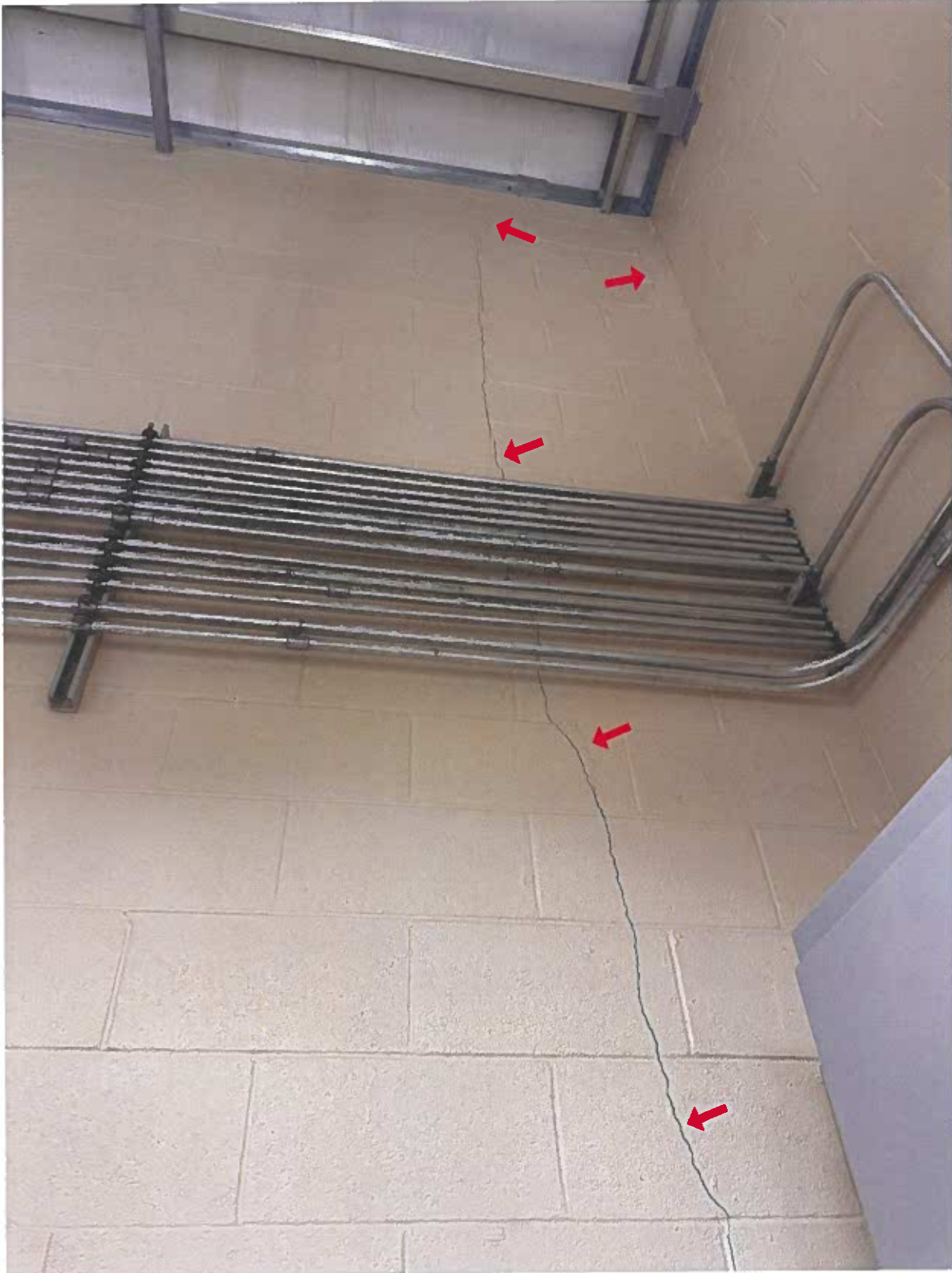
Figure 10: Cracks in masonry wall.
