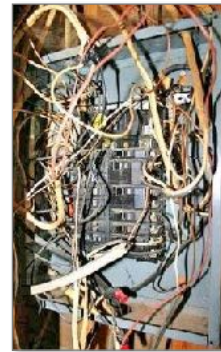
example: Electrical Code violation
