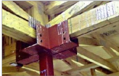
example: Building Code violation
