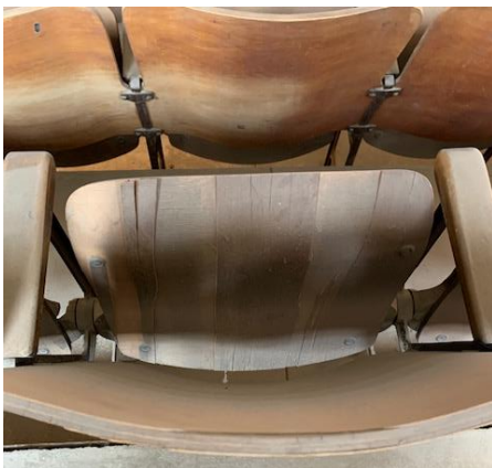
Damaged Wood Veneer
